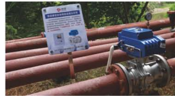
温州仰义东方高尔夫球场 (泄压阀) Wenzhou Yangyi Dongfang Golf Course (pressure relief valve)
