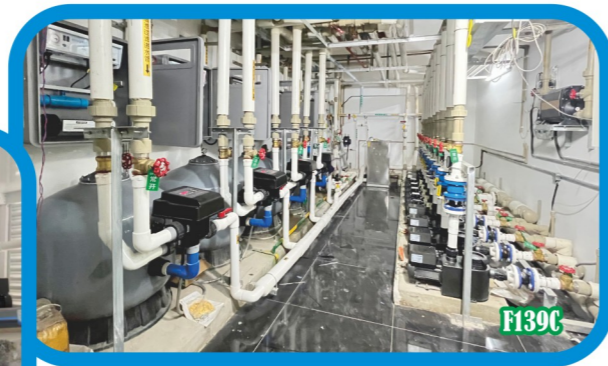
▲广州某高尔夫会所水疗池 Guangzhou Golf Club Spa Pool
