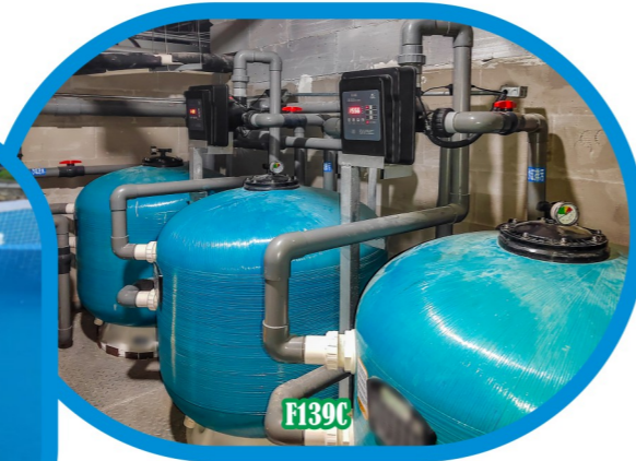
▲山东某泳池公司过滤设备 Shandong Pool Company Filtration Equipment
